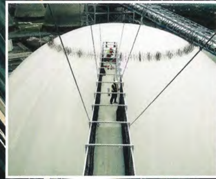
Unusual worked with HTC Tower Cranes and Shepherd Construction on the new biofuel eco-store at Drax power station
