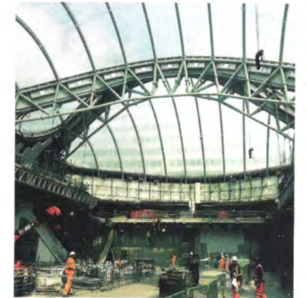
Unusual Rigging built and installed the two suspended work platforms to allow workers reach the atrium roof
